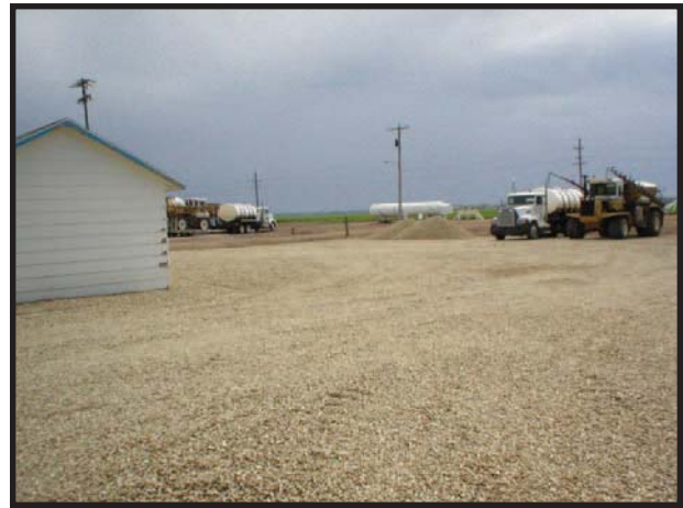
Restoration, such as grading and resurfacing following contaminated soil removal, can be reimbursed through KARB.
