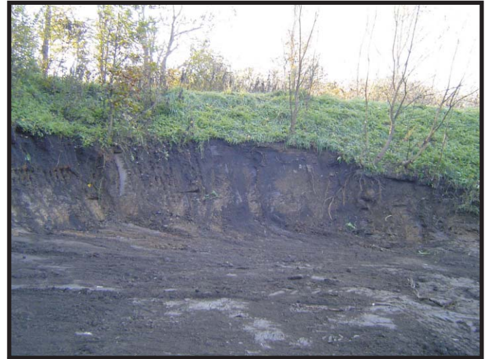
View of berm/backstop for shooting range and area of soil removal. Material removed included soil contaminated with lead, spent bullets, and bullet fragments.
