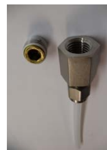
Figure 1. Typical subslab port
