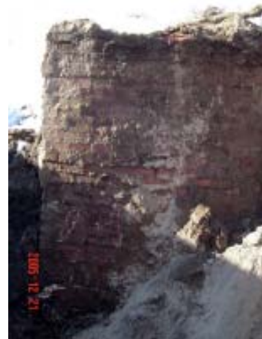
The outside wall of the coal tar well. This kind of brick construction was typical of underground structures at a manufactured gas plant.
