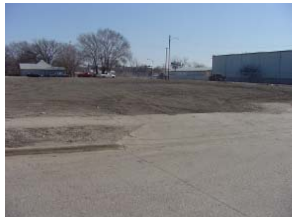
The site after remediation was completed. It can now be redeveloped and put back into use.
