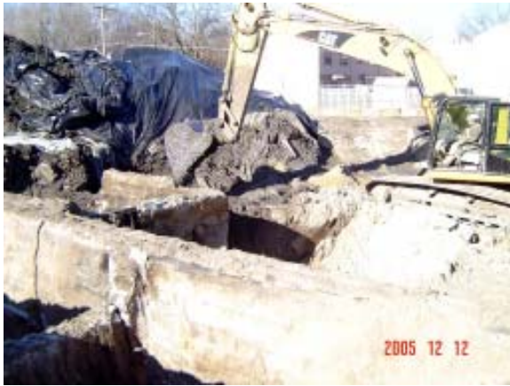
Excavation revealed underground foundations and structures. These were left in place when clean fill was installed.
